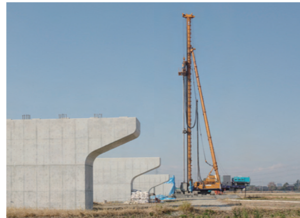
The low displacement construction method makes construction work possible in proximity to existing buildings.
